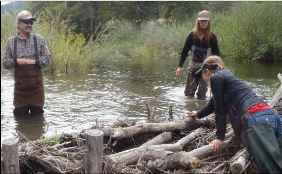
Above: Sugar Creek BDA after construction created an upstream pool. Credit: USFWS
